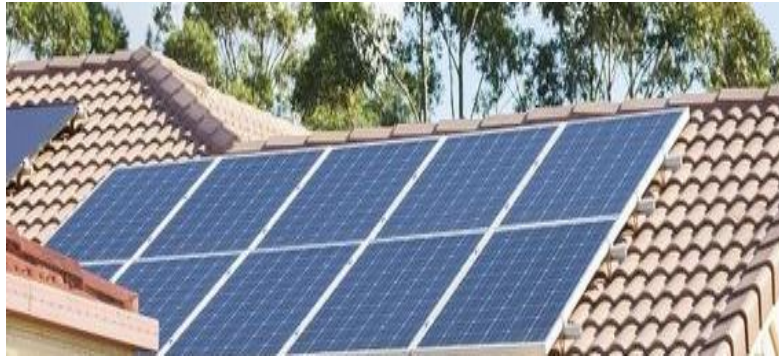
Figure 1. Roof-installed PV solar panels
